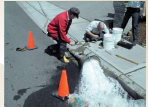
To improve water quality, Bellevue flushes about 20 percent of its system each year.
